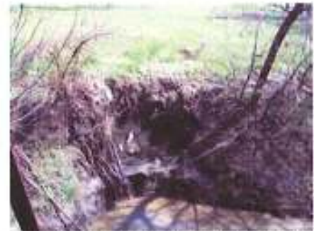
Figure 9: Photograph of Cross Creek bank erosion. Source: Brad Hus.
