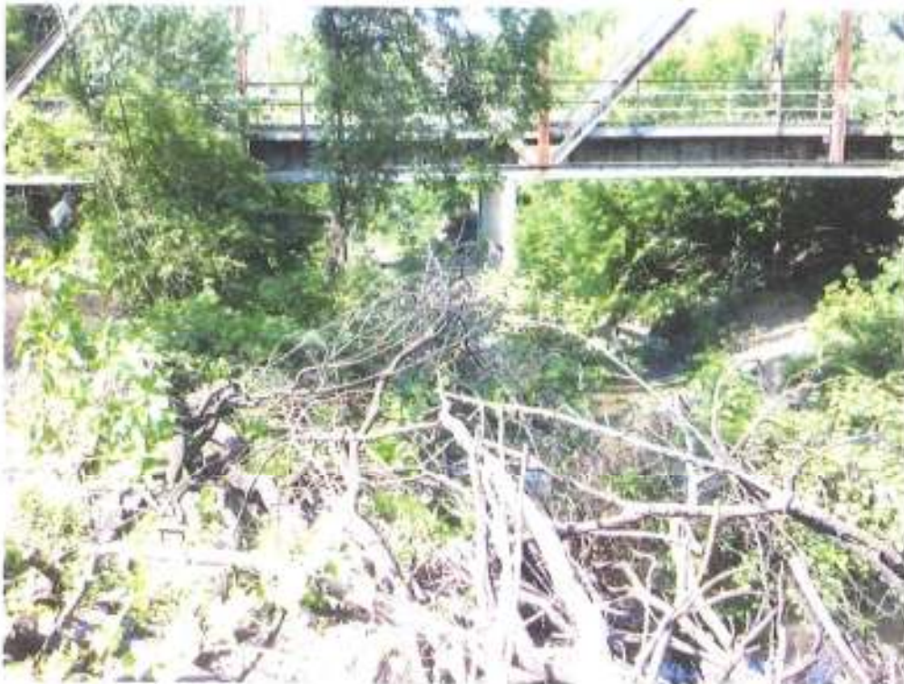
FIGURE 9: ABANDONED 42ND TERRACE BRIDGE
