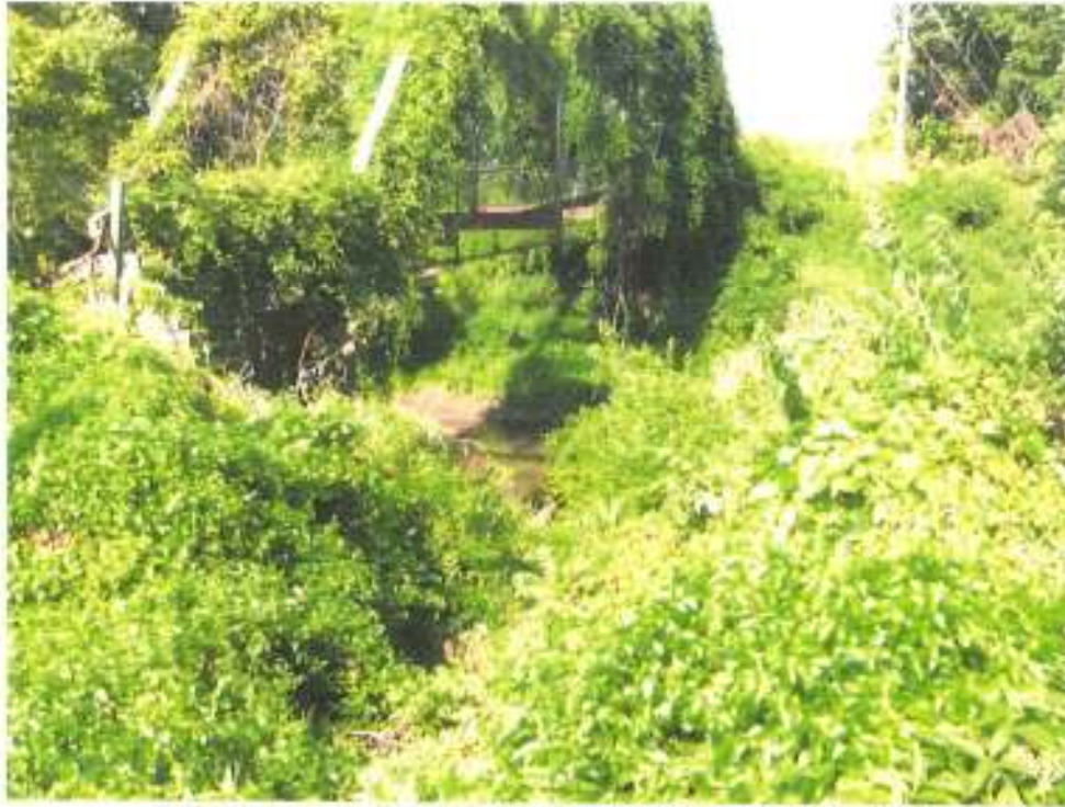
FIGURE 8: ABANDONED 46TH STREET BRIDGE
